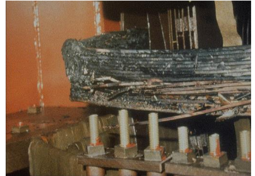
Example of a transformer coil that overheated.
