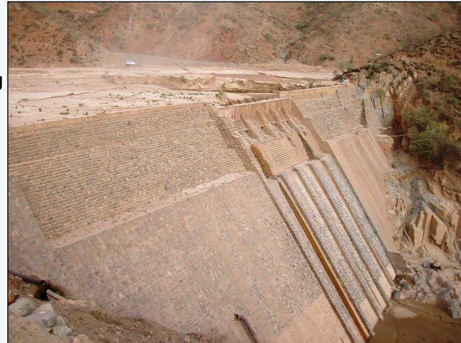
Completely silted Denadai Dam in Eritrea (De Vito, n.d.)
