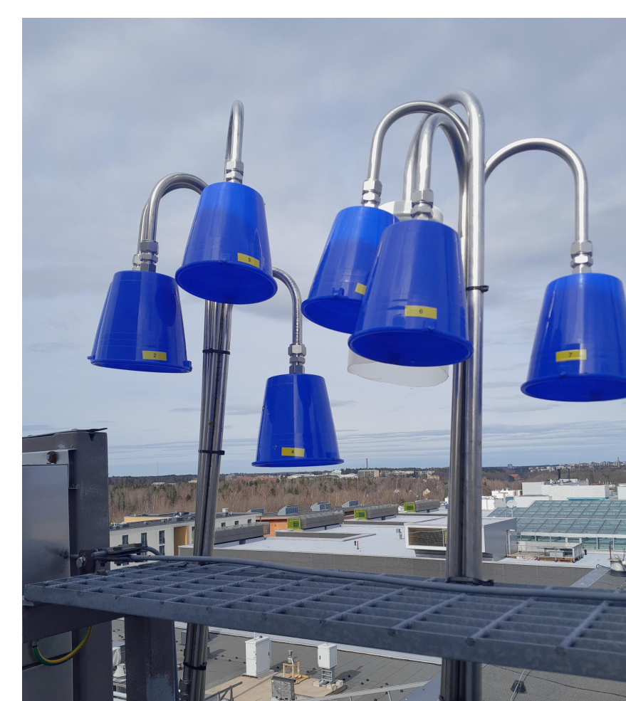
(b) Filter inlets
