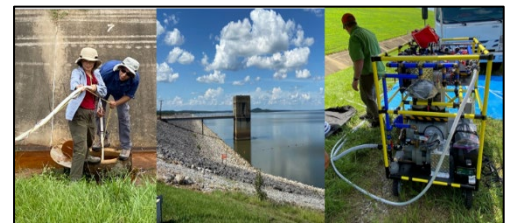
Figure 2: Engineer and scientist deploying hose into relief well at the toe ditch for treatment of encrusted biofilm.
