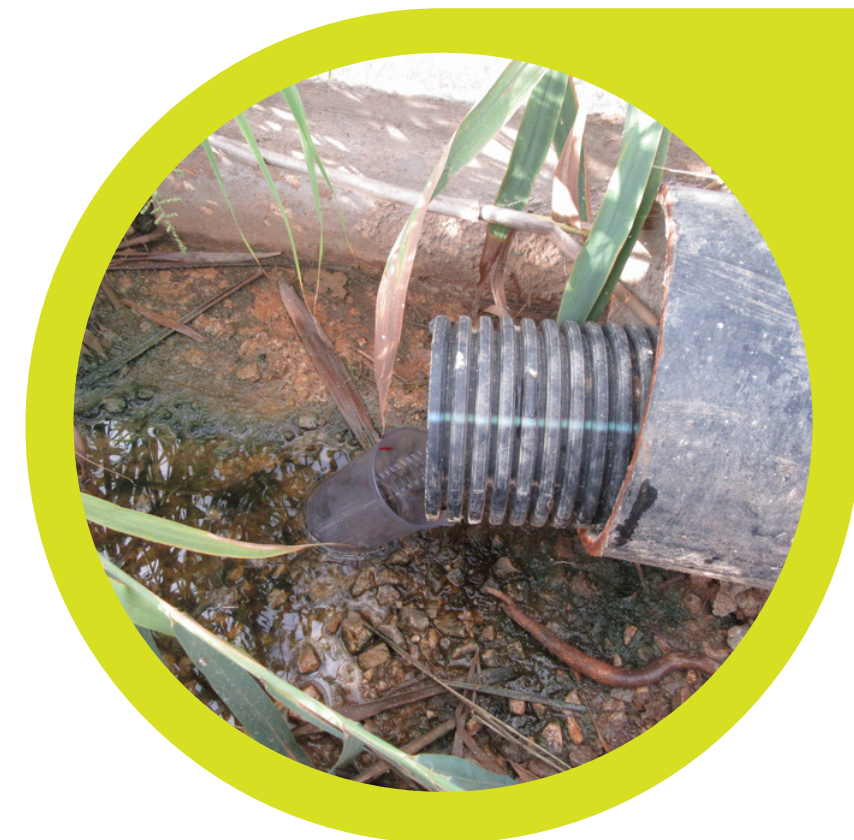
Subsurface drainage pipe outlet
