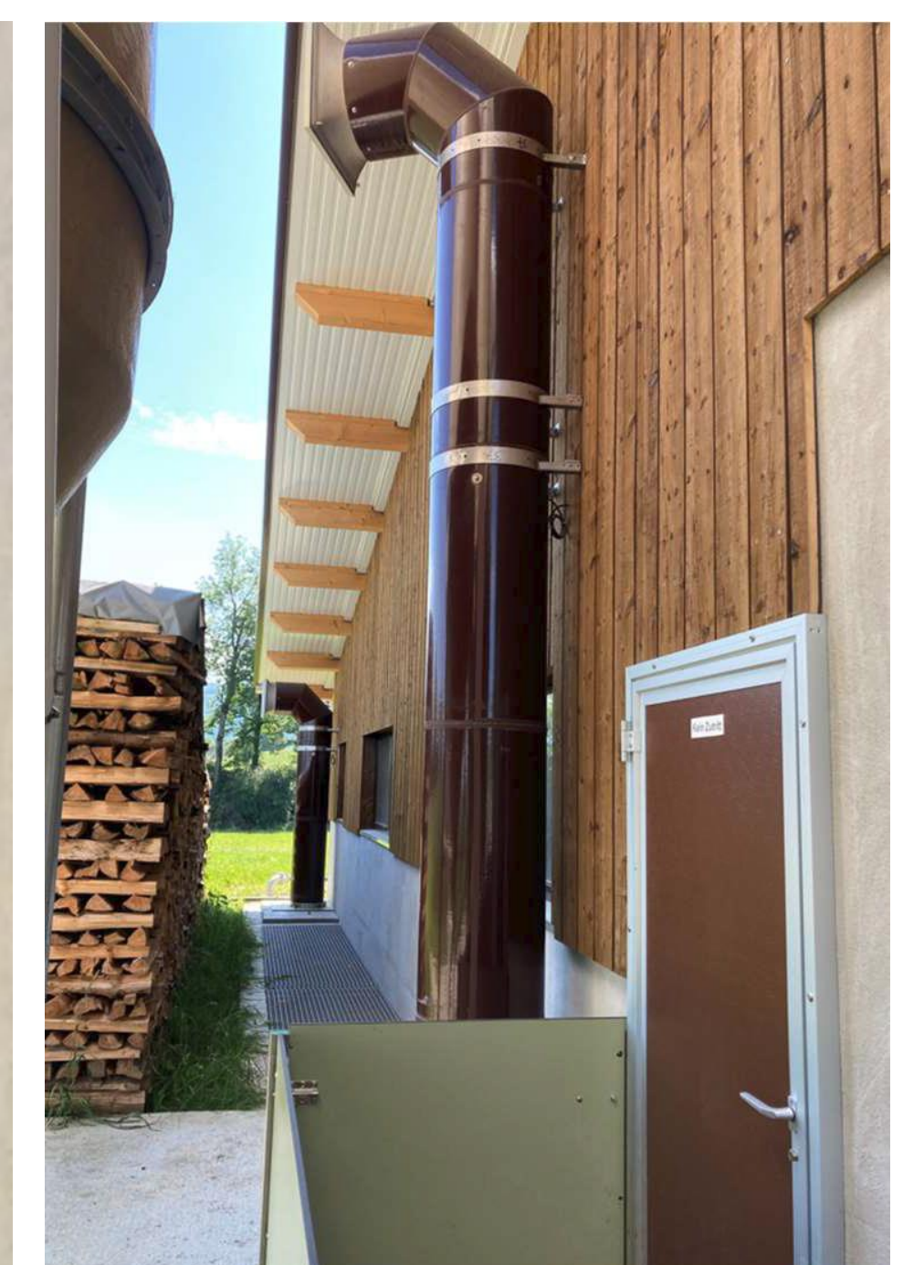
Exhaust duct for channel ventilation
