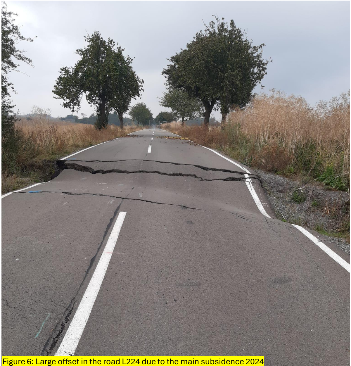
Figure 6: Current cracking on the road L224 in the context of the main subsidence 2024
