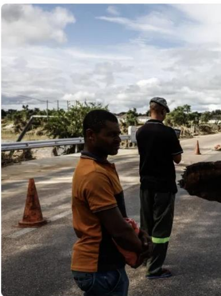
Onlookers inspect damage to the bridge crossing the Ga-Selati river following heavy rains over much of the Limpopo Province, South Africa.
