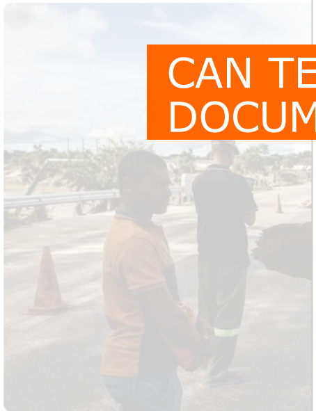
Onlookers inspect damage to the bridge crossing the Ga-Selati following heavy rains over much of the Limpopo Province, South Africa.
