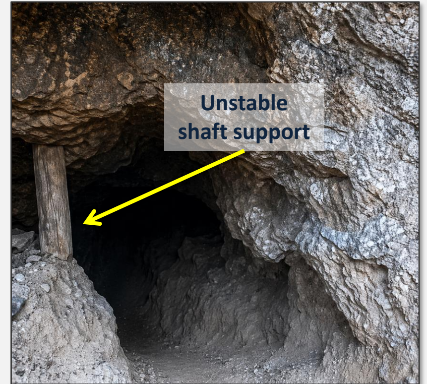
Figure 8: Unstable shaft support.
