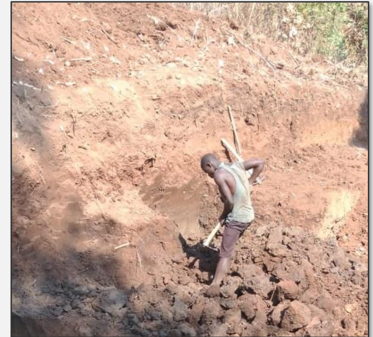
Figure 9: Excavation instability and unsafe conditions in artisanal mining.
