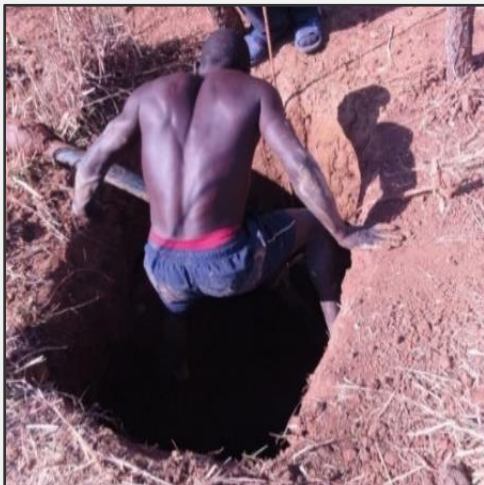
Figure 12: Manual access to underground pits without structural support.
